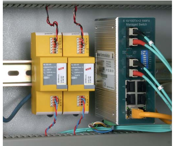
Protection of the loudspeaker outputs of a voice alarm system.
