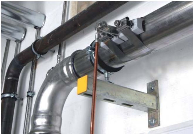
Installed at a StSt pipe
