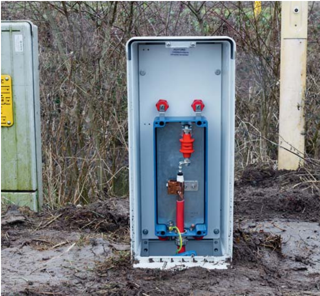
Coaxial connection of the Ex isolating spark gap for protecting buried insulating joints
