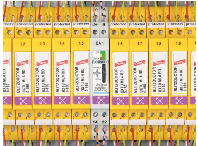
Installed DEHNrecord condition monitoring system
