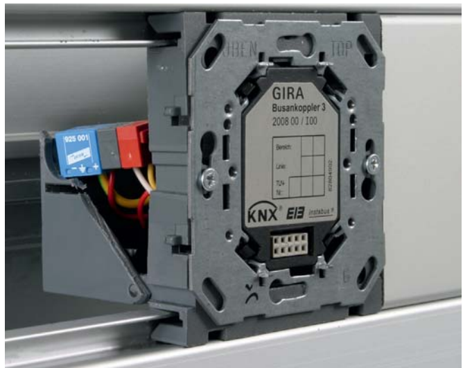
Protection of a KNX bus coupling unit by means of a BUSector surge arrester mounted on a bus terminal in the mounting panel of a cable duct
